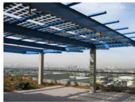
Optima Biltmore Towers Solar Array by PerfectPower Inc.
