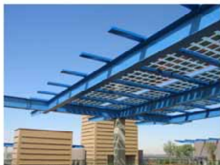
Optima Biltmore Towers Solar Array by PerfectPower Inc.
